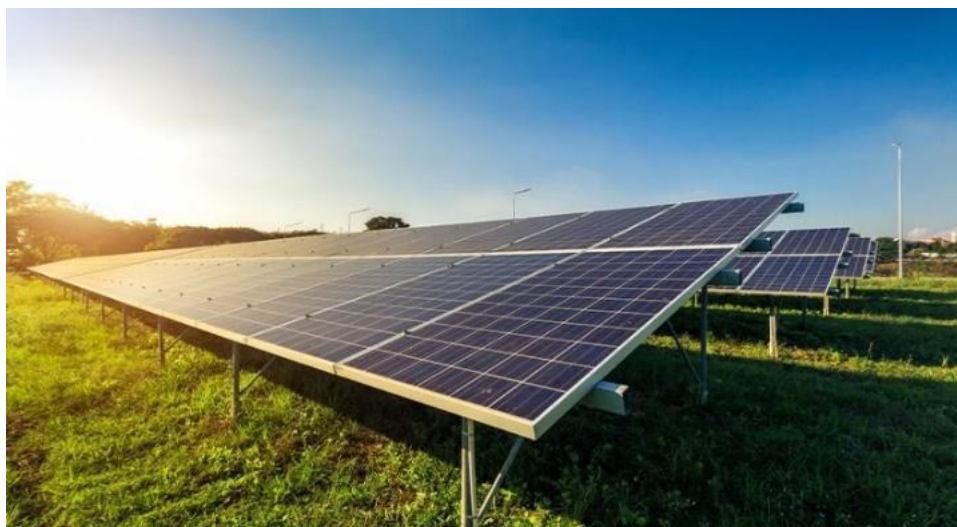
Figure 1. Solar Panel System.
